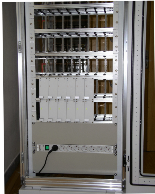
SE-RM1 Surface switchboard with 6 SAZ-T1 seismic-acoustic boards and 6 SE-S1 supply boards
