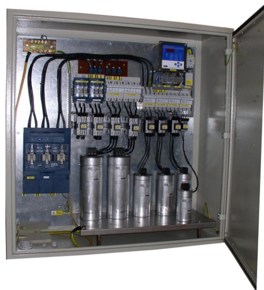
Switchboard cabinet RK1
